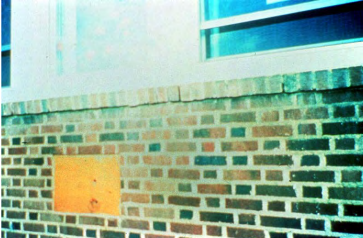
Figure 11 Plywood covering the outdoor air intake for a classroom. Applied during the oil embargoes of the 1970s, the classroom remained under-ventilated until the mid 1980s.
