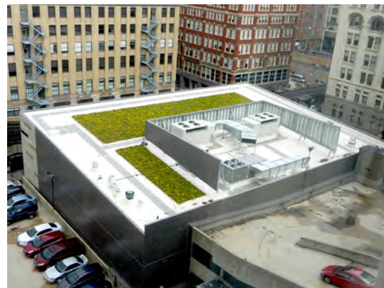
Figure 7.15. A vegetative roof system with paths that could be used for access and ventilation.
