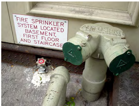
Figure 8.9. A sign indicating the areas covered by the sprinkler system that is fed by the FDC shown.
