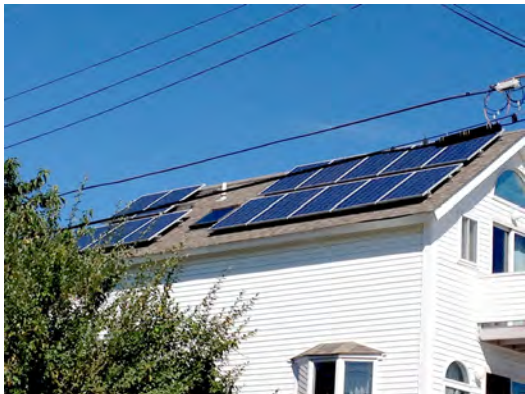
Figure 7.14. Photovoltaic panels on a roof.
