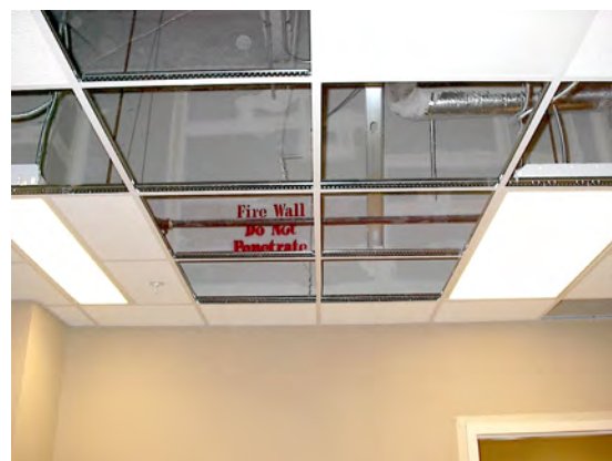
Figure 13.14. A “Do Not Penetrate” sign stenciled on a fire barrier wall above a suspended ceiling. The sign is intended to warn workers modifying the utilities located in the space above the ceiling.
