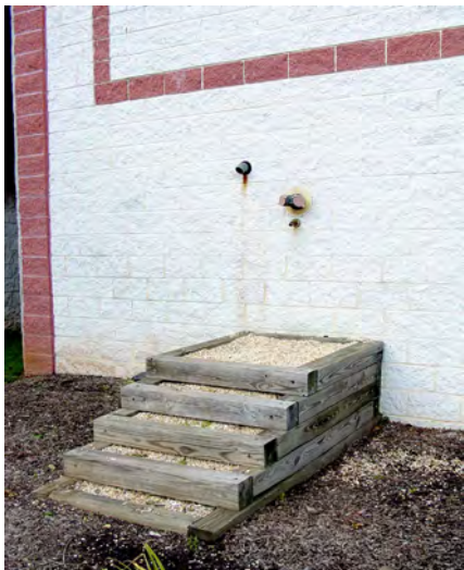
Figure 10.12. A platform built up to reach an FDC. This creates an unnecessary fall hazard.
