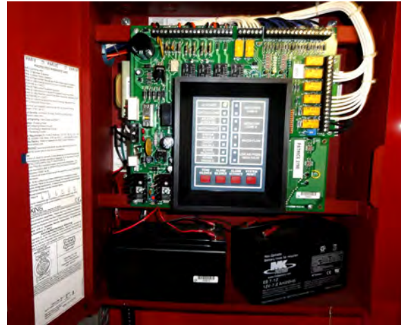
Figure 11.1. A basic fire alarm control panel with its door open, showing the wiring and the batteries for backup power. The controls and indicator lights in the center are visible when the panel door is closed and locked.
