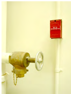
Figure 12.8. A firefighter emergency power outlet next to a standpipe fire hose connection.
