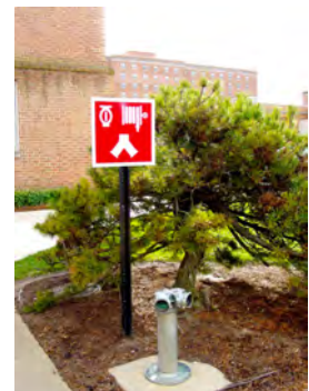
Figure 10.14. An FDC sign with the NFPA 170 symbols for both sprinkler and standpipe systems.
