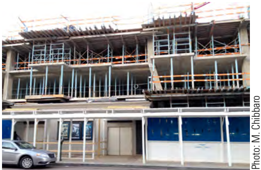
Figure 13.12. A typical 4 ft.-wide temporary walkway (painted white) over a sidewalk adjacent to a construction site. The wide span between posts accommodates the double exit doors (shown in the center), which serve an occupied cinema.
