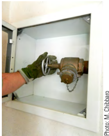
Figure 9.13. A FHC in a cabinet being checked by an inspector wearing a firefighting glove.
