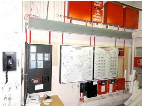
Figure 11.15. The inside of a fire command center.
