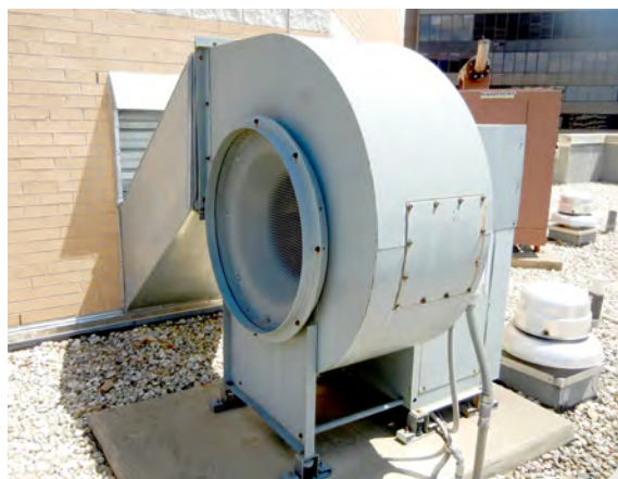
Figure 12.12. A stair pressurization fan.
