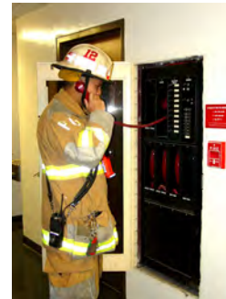
Figure 11.13. A fire officer speaking into the main handset at the control panel for a fire department communication system. This panel also houses the portable handsets used by firefighters at remote jacks.
